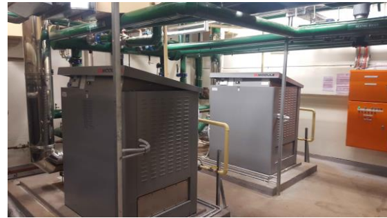
Two new 550kW condensing boilers
