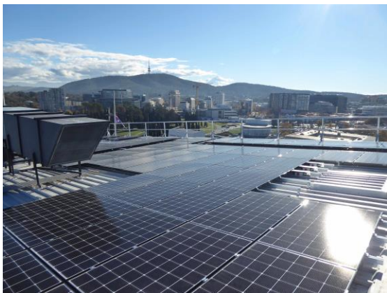
The PV system maximised the available roof space whilst maintaining service access
